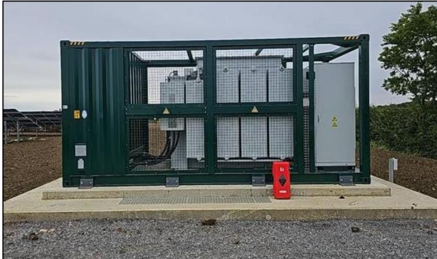
Plate 1.3: Typical outdoor transformer
