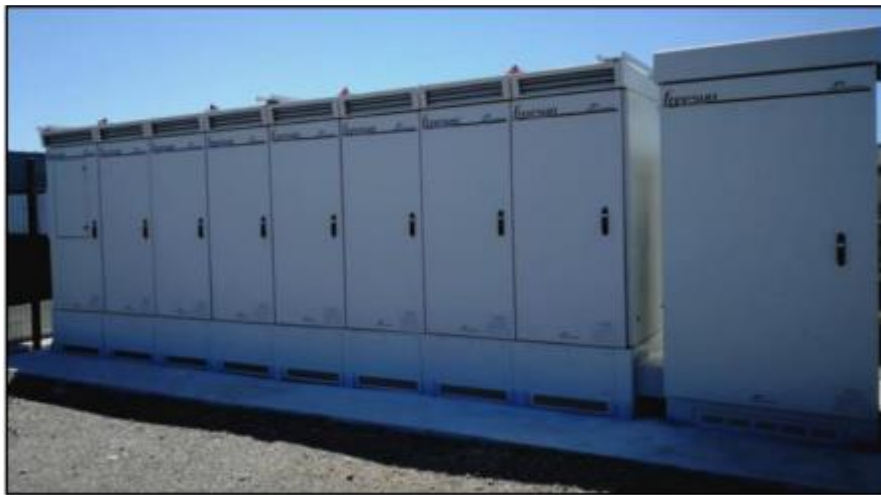
Plate 3.2 Typical Centralised Inverter
