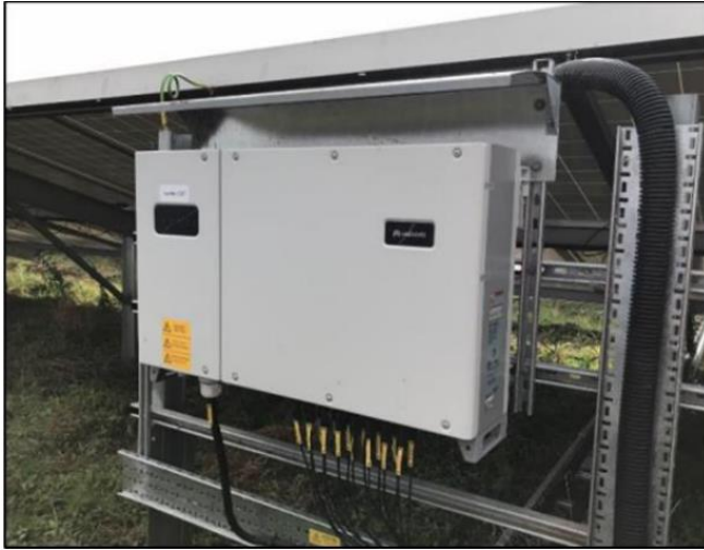
Plate 3.1 Typical String Inverter
